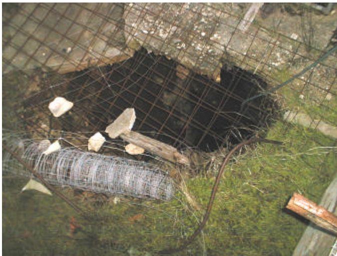
Y2 Entrance and Collapse.
