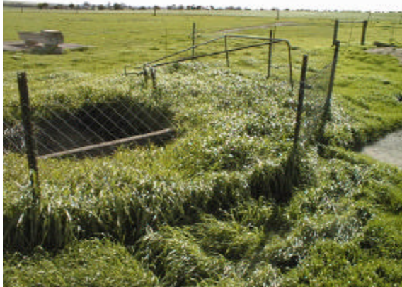
Y1 Collapse Pit.
