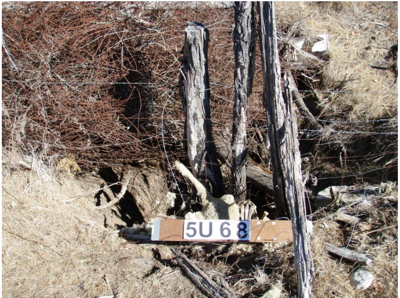
U68 rubbish-filled pipe with dead sheep
