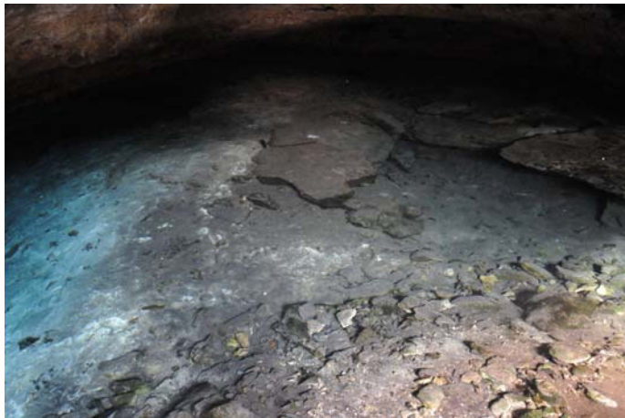
Figure 9: Roof collapse on top of rock pile/boulders, showing subsequent roof collapses (NRS)
