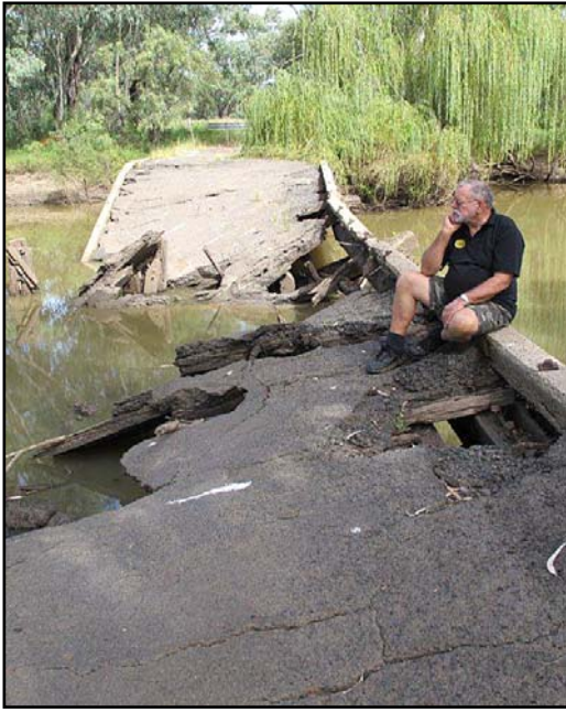
Damaged Bridge at Augathella
