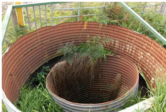
The two tanks. Note undermining of the outer tank on the left and right.
