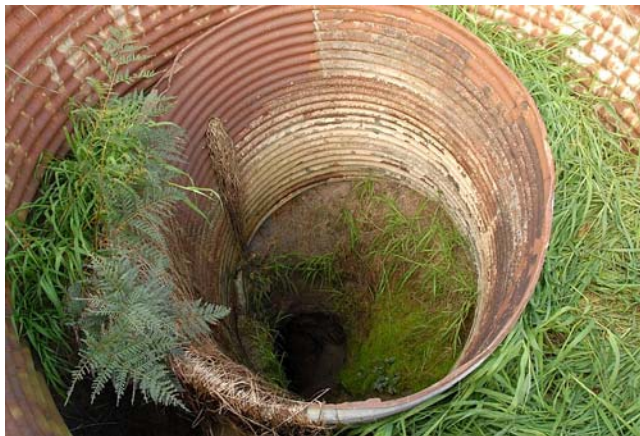
The two tanks and top of the solution pipe. The inner tank is undermined at the left and bottom right of the picture.
