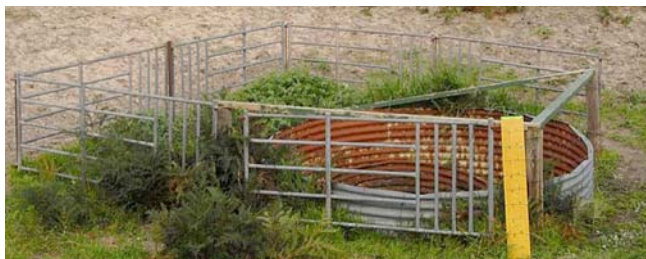
The cave entrance prior to the 9 th of September. Note the two fences and tanks and the collapsed wooden railing. The yellow plank is one metre long.
